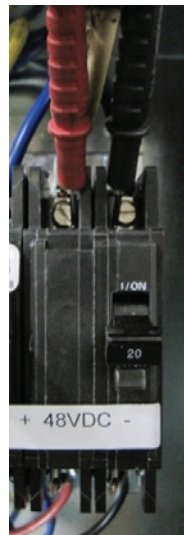
DC Field Voltage Connections at Top of the Breaker
