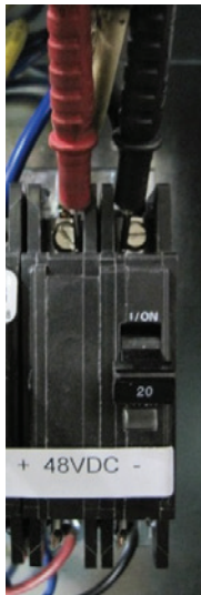
DC Field Voltage Connections at Top of the Breaker
