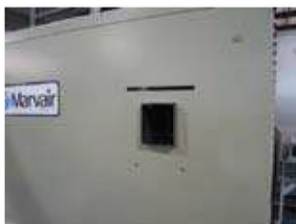
VENT HOOD OPENING
